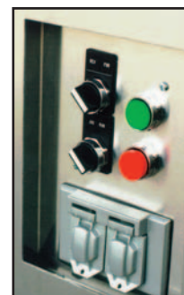
Push Button Controls
